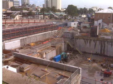
3CC concrete pile wall (top left), Diaphragm wall section (right) and CALTITE "composite" slab.
